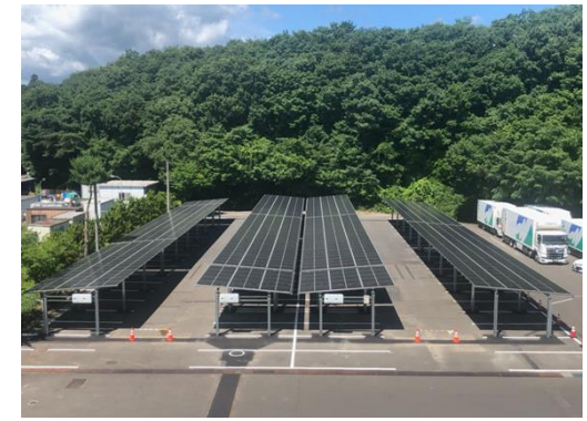
Solar panels on the carports for employees
