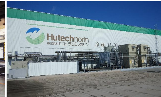
Installed refrigerators with natural refrigerants
