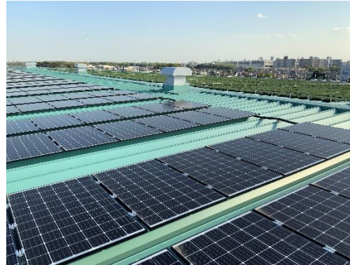
Solar panels on the rooftop of facilities
